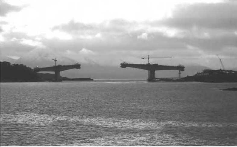
2. The end of an island? Bridge to the Isle of Skye under construction, Scotland, UK (source author, 1995)
